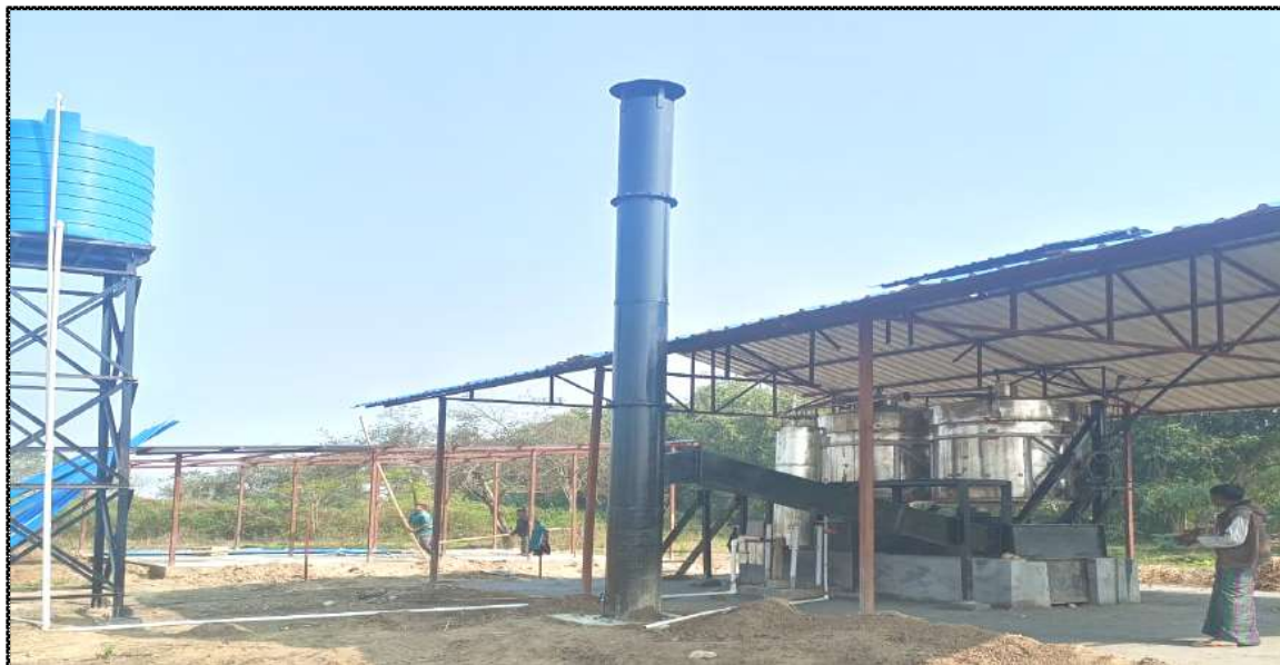
One ton capacity hydro-steam distillation unit established at Nampong Village, Namsai district, Arunachal Pradesh
